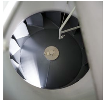
Water injection to avoid/reduce the build-up of deposits
