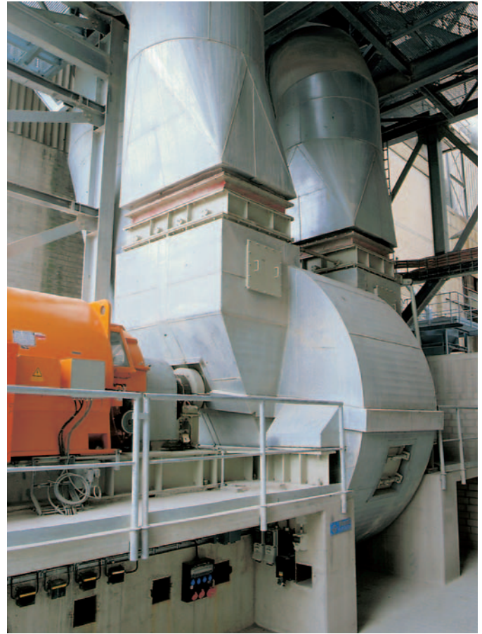
Figure 7: Circulated air fan for cement mill
