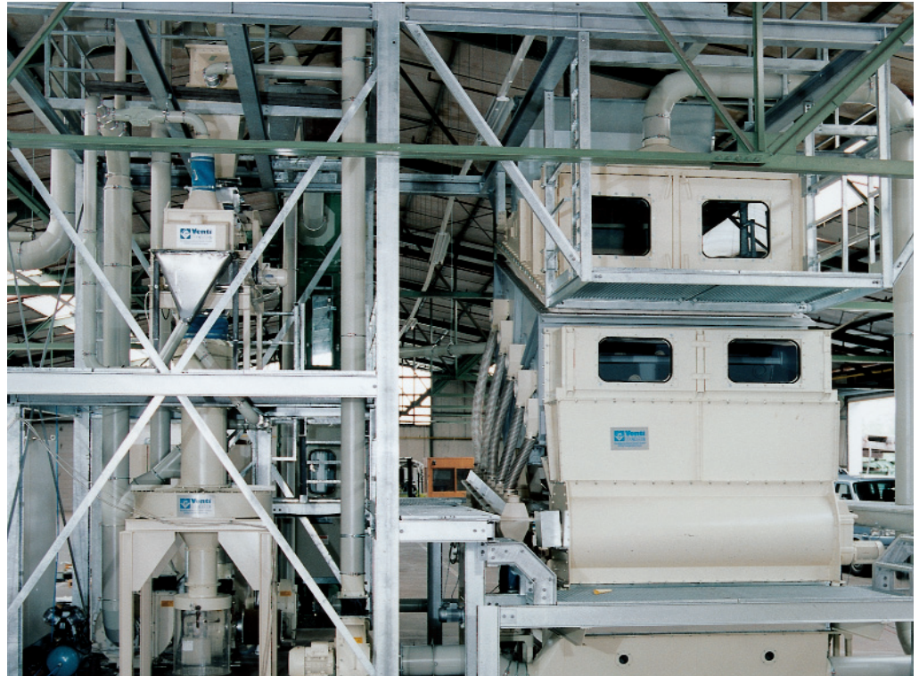
Overall view of plant layout
